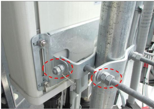
Loose mounting brackets
